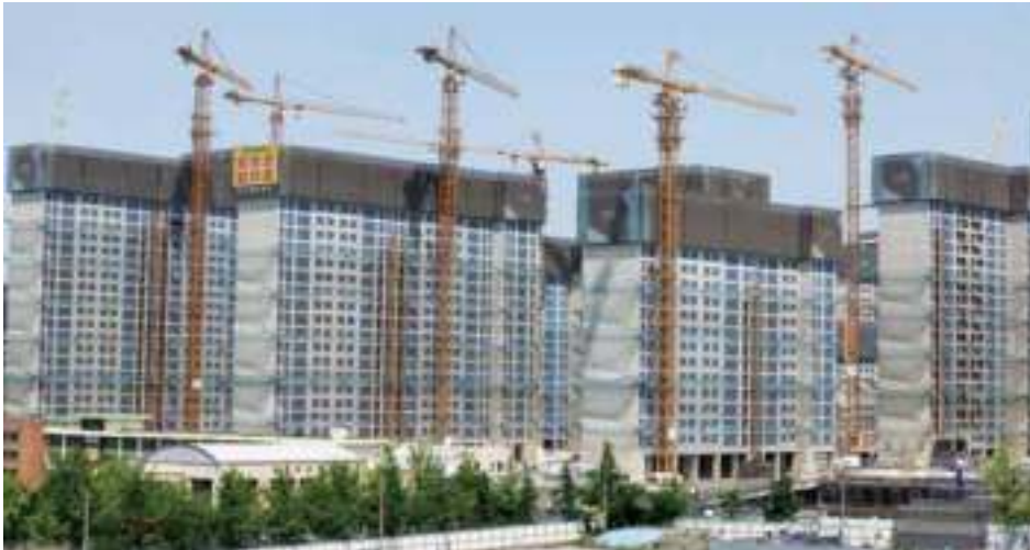
Dunchon Apartments is a redevelopment project consisting of 85 residential towers situated at the prominent site of the old Olympic Village in Seoul
